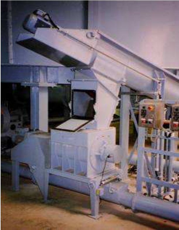
Pneumatic Feeding System, Rotary sluice
